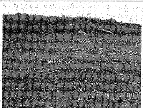
Photo 2. Exposed waste at the northeastern side of the Landfill.
