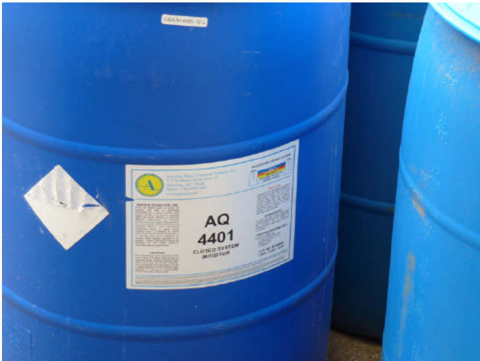
Chemical Drums near the Solar Thermal Equipment.
