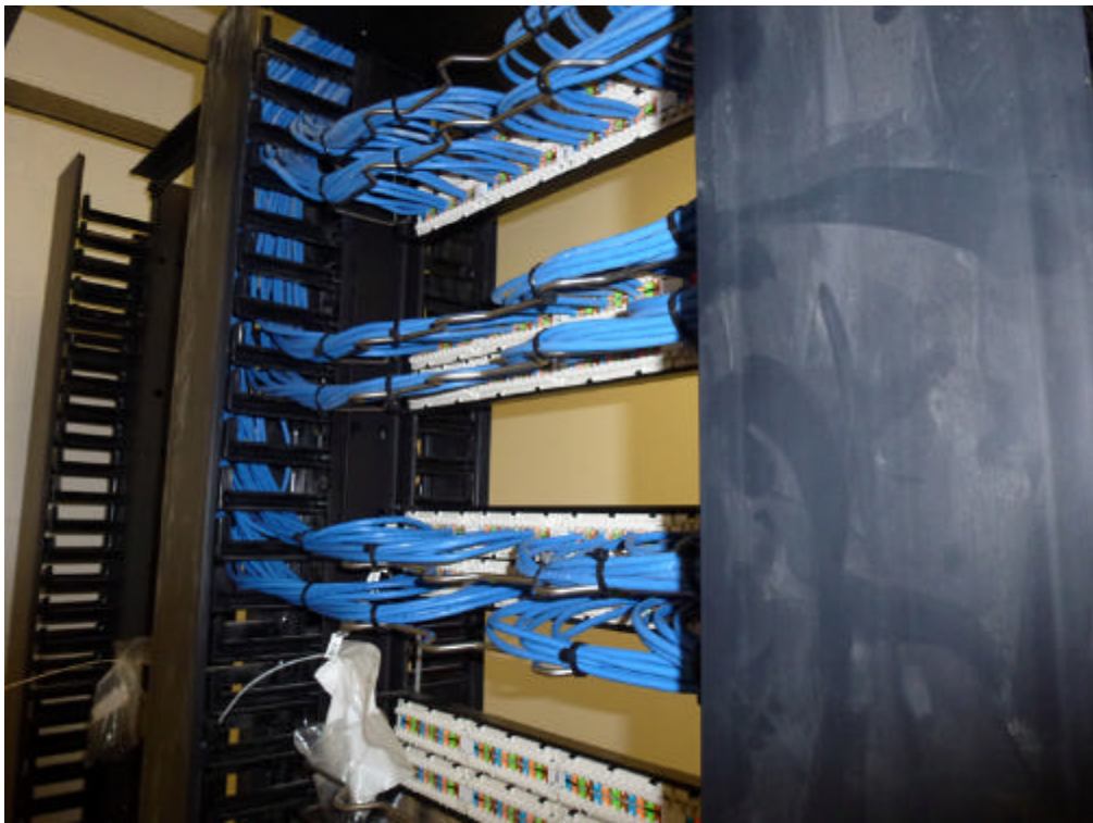
Rear of panel.
