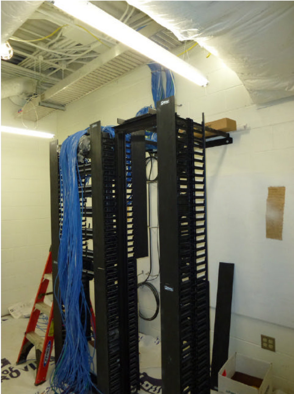
Rack on the second floor.
