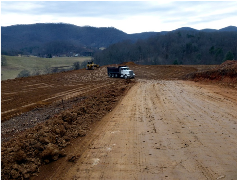
One of the trucks returning from dumping the dirt and going for another load.
