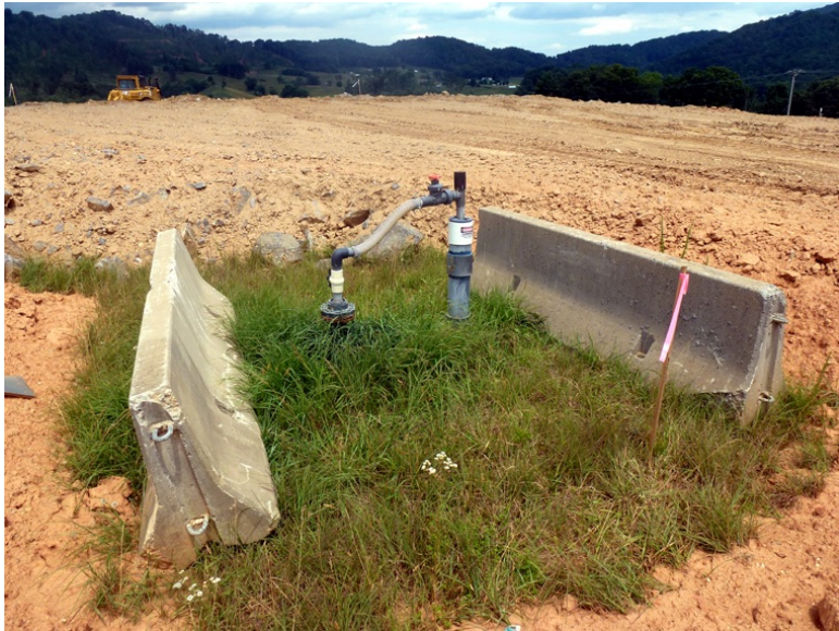
This is one of the multiple wells on top of the landfill. Obviously, these will have to have extension risers installed to elevate them to a new ground level.
