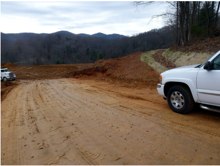
Perspective view looking down the road, landfill is up to the right.
