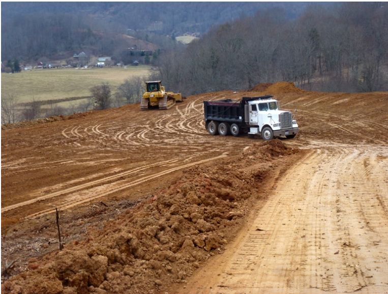
Zoom shot. When we returned on 6/29/2015, this area had been widened, had drainage installed around the outside perimeter, and planted with grass. It did not appear that any of this dirt was being used for placing on the top of the landfill.
