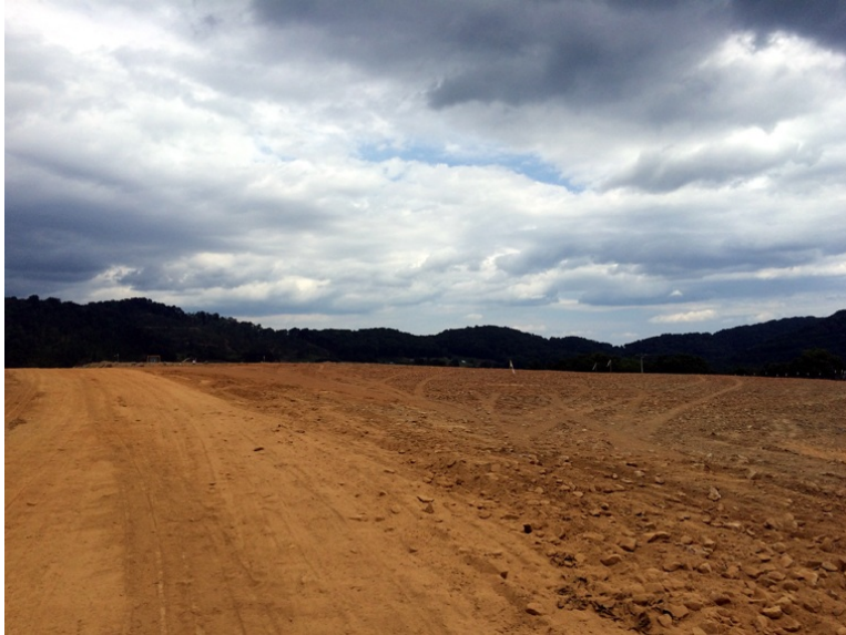
This is the entrance to the top of the landfill off the perimeter road.
