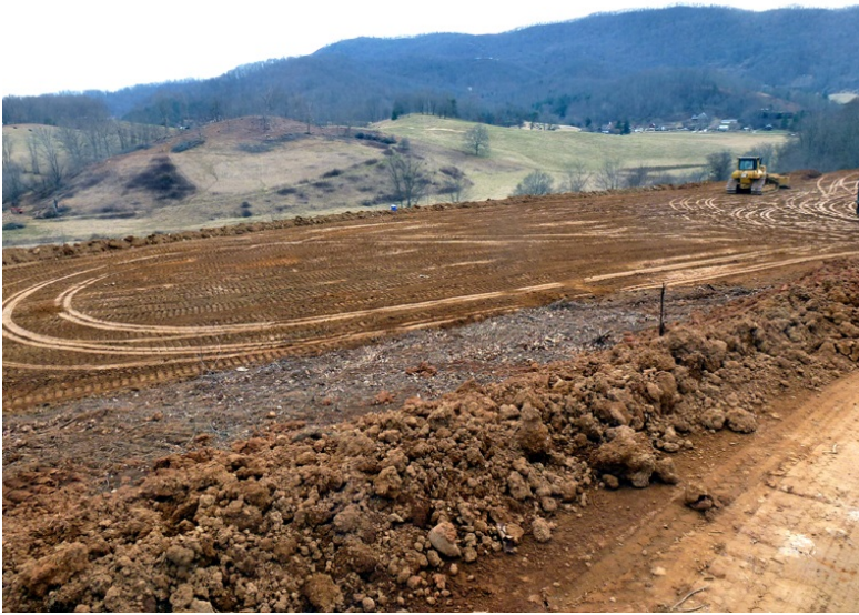
After going down this little road, dirt was being leveled with a bulldozer.
