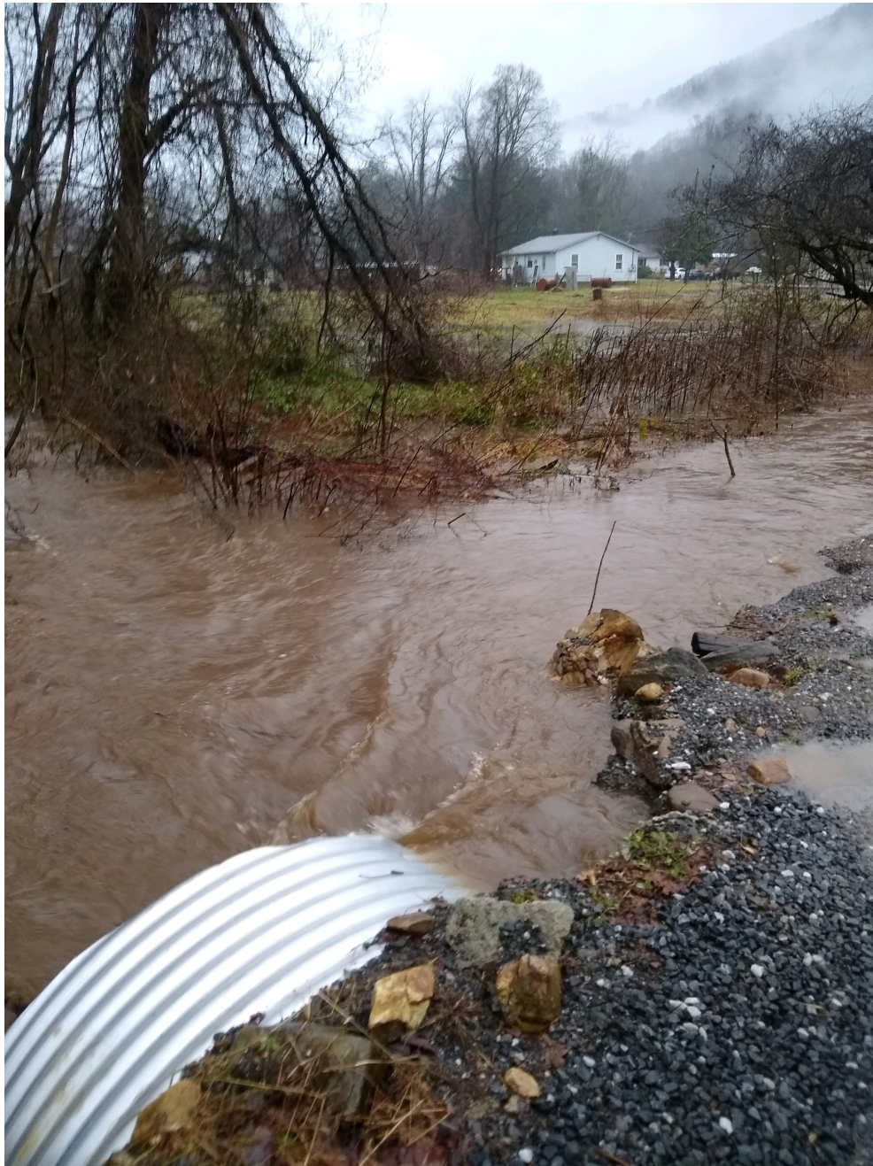
This is the (overworked) existing culvert. Water going to the right is heading over to Charley's lawn. This view is looking from the culvert back to Allens Creek Road, where the grocery store was demolished.
