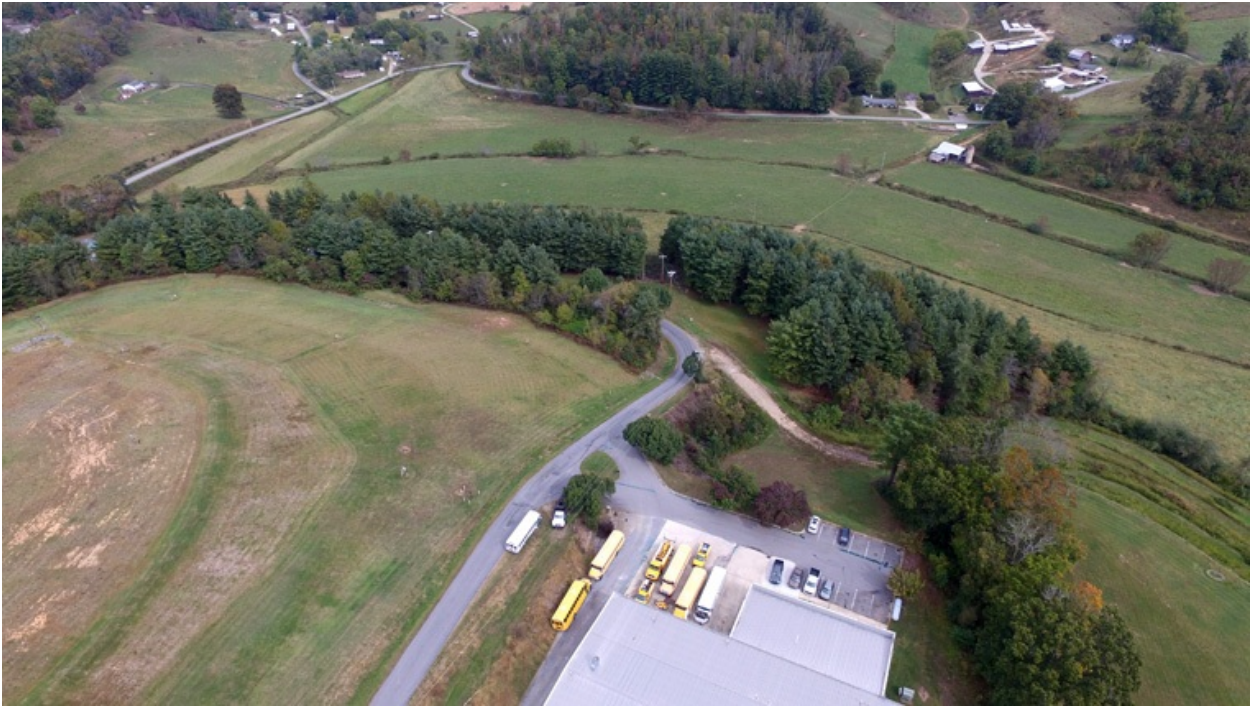
This photo is from a higher elevation, and shows the area of stockpiled dirt from collected from the Old Walmart DOT exchange. It is seen at the lower right corner of the photo. This is the dirt that will grade the land before the cap, and then cover the cap.
