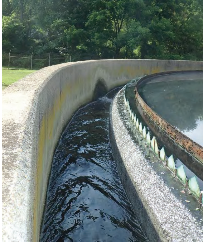
Figure 3. Annular drainage trough at primary clarifier.
