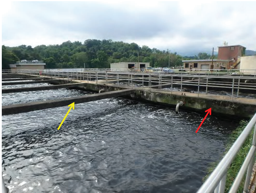
Figure 8. Aeration basin. Walkway (red arrow) tops interior wall that separates chambers. Horizontal braces (yellow arrow) provide lateral stability to walls.
