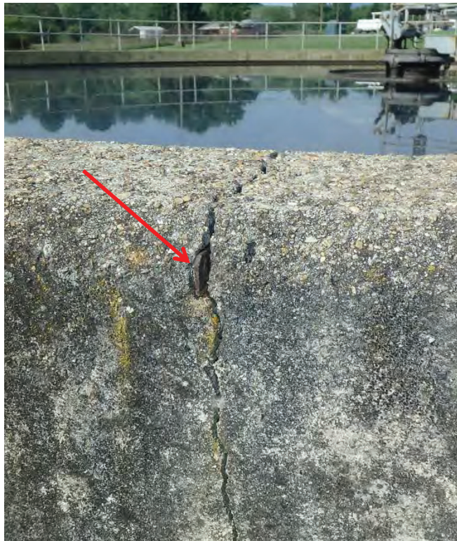
Figure 4. Typical crack at primary clarifier. Red arrow indicates metal form tie.
