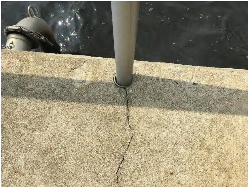
Figure 12. Freeze-thaw cracking at guardrail post penetration.
