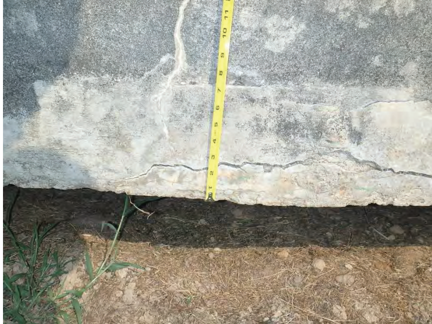
Figure 7. Severely delaminated concrete at base of primary clarifier.
