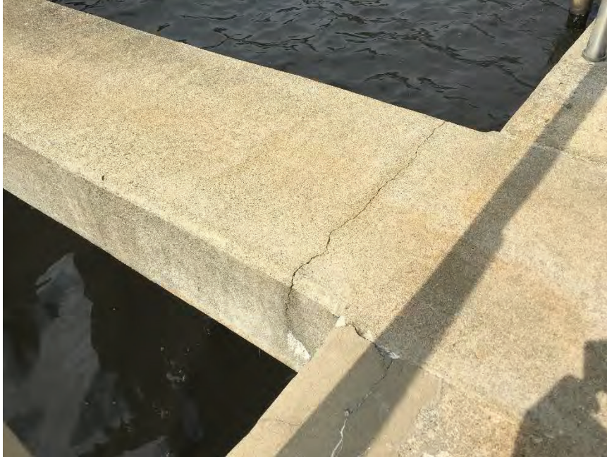
Figure 11. Minor flexural crack and delaminating concrete at horizontal brace.
