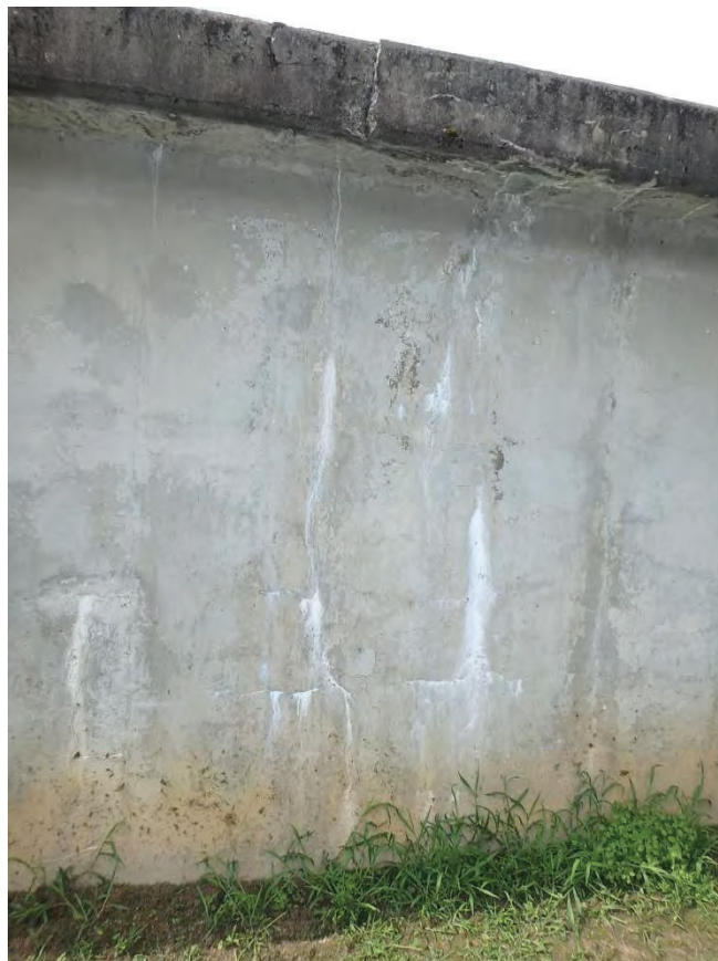
Figure 10. Typical cracks with efflorescence at north perimeter wall of aeration basin
