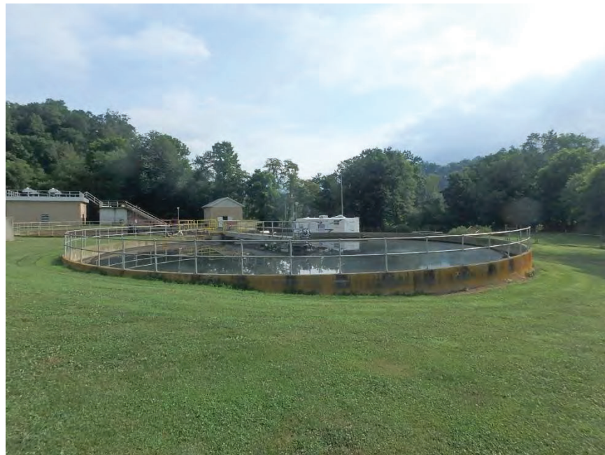
Figure 2. Concrete at primary clarifier is stained but in generally good condition.
