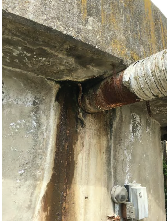
Figure 17. Leaking pipe at north-most sludge thickener.
