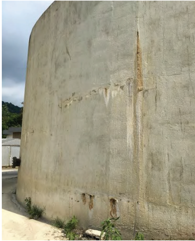
Figure 15. Cracks with efflorescence and corrosion staining at digester.
