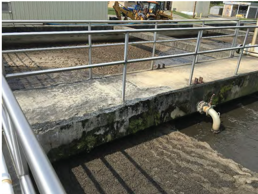
Figure 14. Widespread spalling and raveling of concrete at aeration basin walkway.
