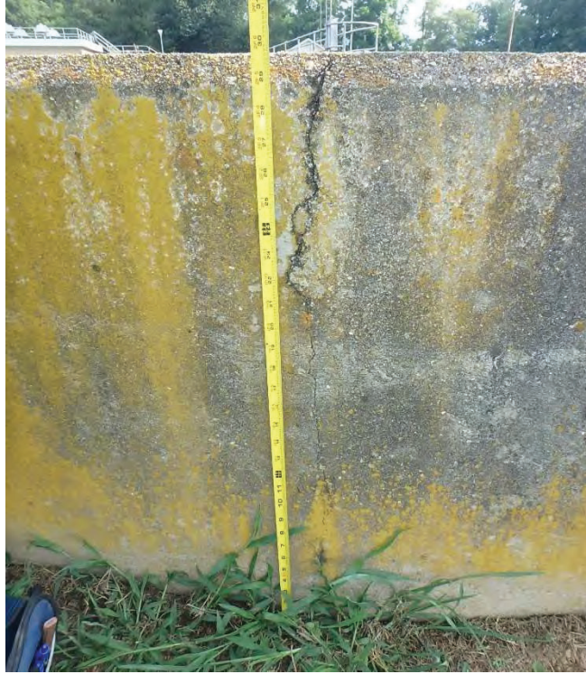
Figure 5. Crack at primary clarifier with minor leakage.
