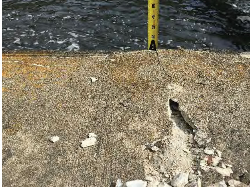
Figure 13. Localized delaminations and spalling at aeration basin walkway.
