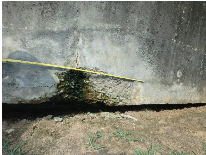
Figure 6. Spalled concrete coincident with leaking crack at primary clarifier.
